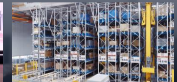
Commissioning the intelligent three-dimensional warehouse system
